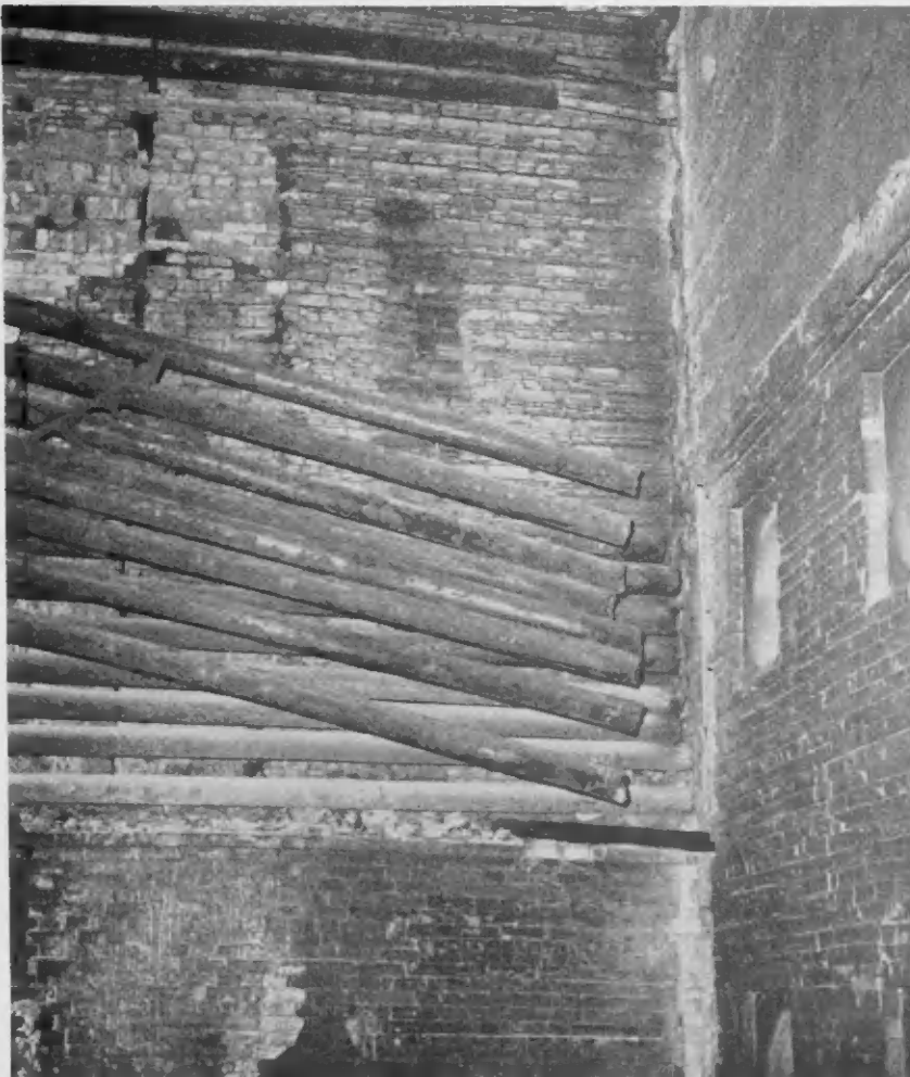
THE INSIDE of the furnace on No. 9 Visbreaker looks like this before the back brick wall is dismantled. Pipes in the convection section hang down just before being pulled. A new wall with bracing will replace the back wall. A bulldozer operator, right, winches out a tube bundle with the help of a derrick, not shown.
